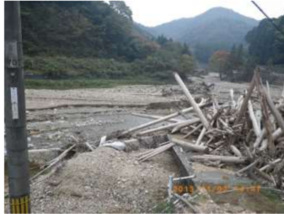
Figure 1. Woody debris accumulation at the bridge.
